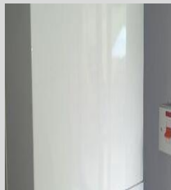
Typical combi on site – RWH5
